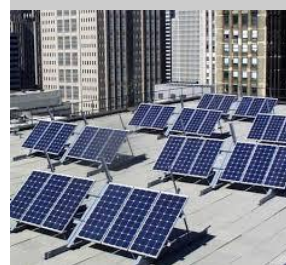
Panels tilted at an angle to the roof- Not exempt
